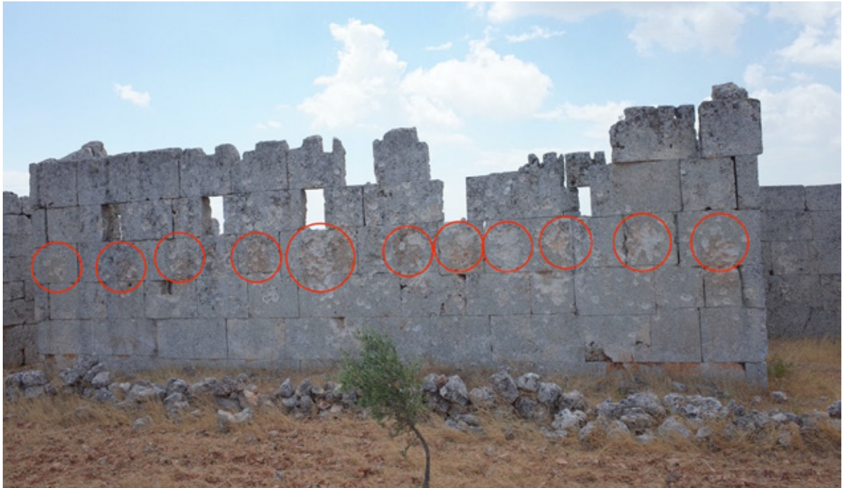
Figure 8 Traces of munitions fire on the house-church's north-side wall
