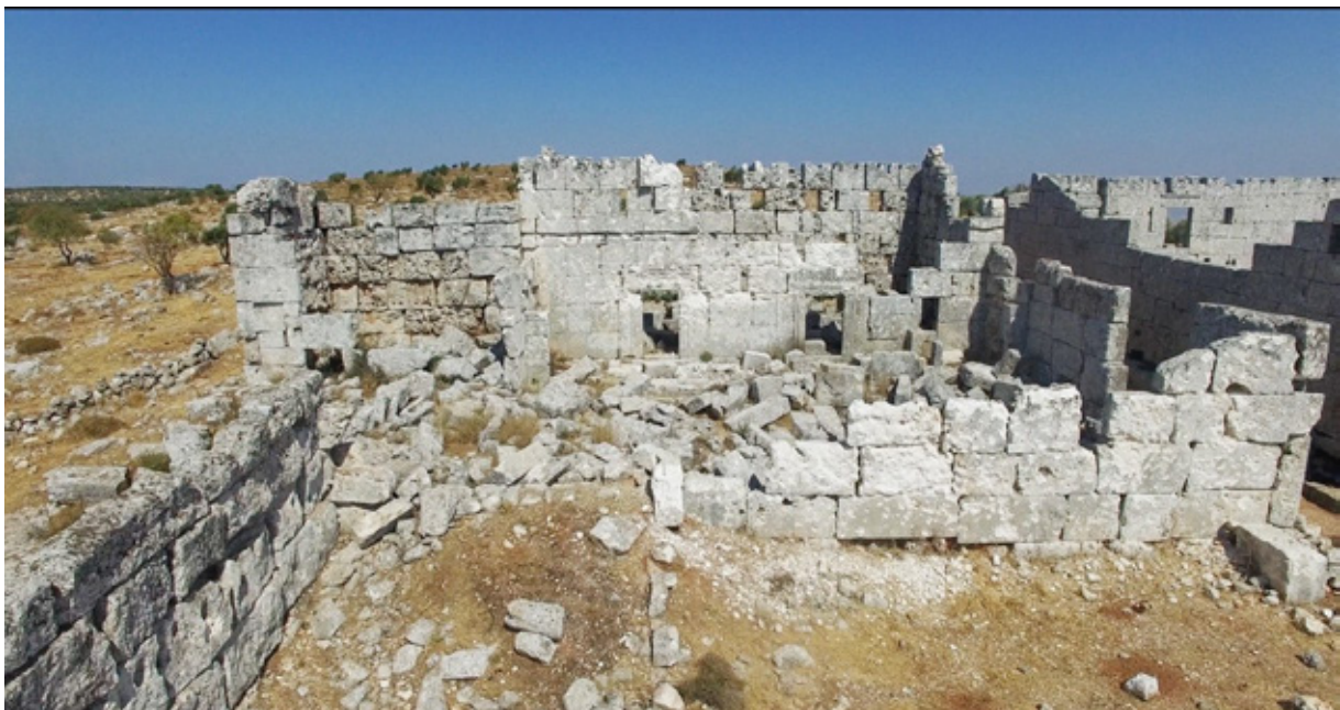
Figure 7 Traces of munitions fire on the south-side walls of the southern courtyard and altar's hall
