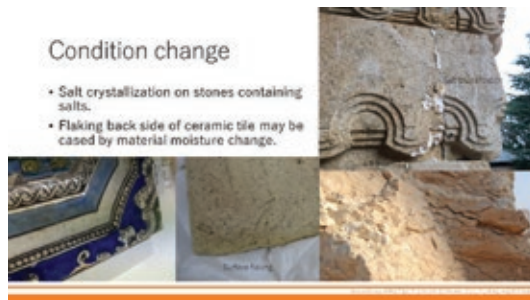
Figure 7 Flaking of the tiles and salt crystallization of stones
