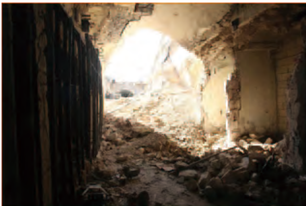
Fig. 3 Aleppo historic souk burns as clashes continues in Old City of Aleppo.
